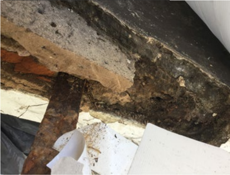
Close Up of Remains of Balcony Structure
